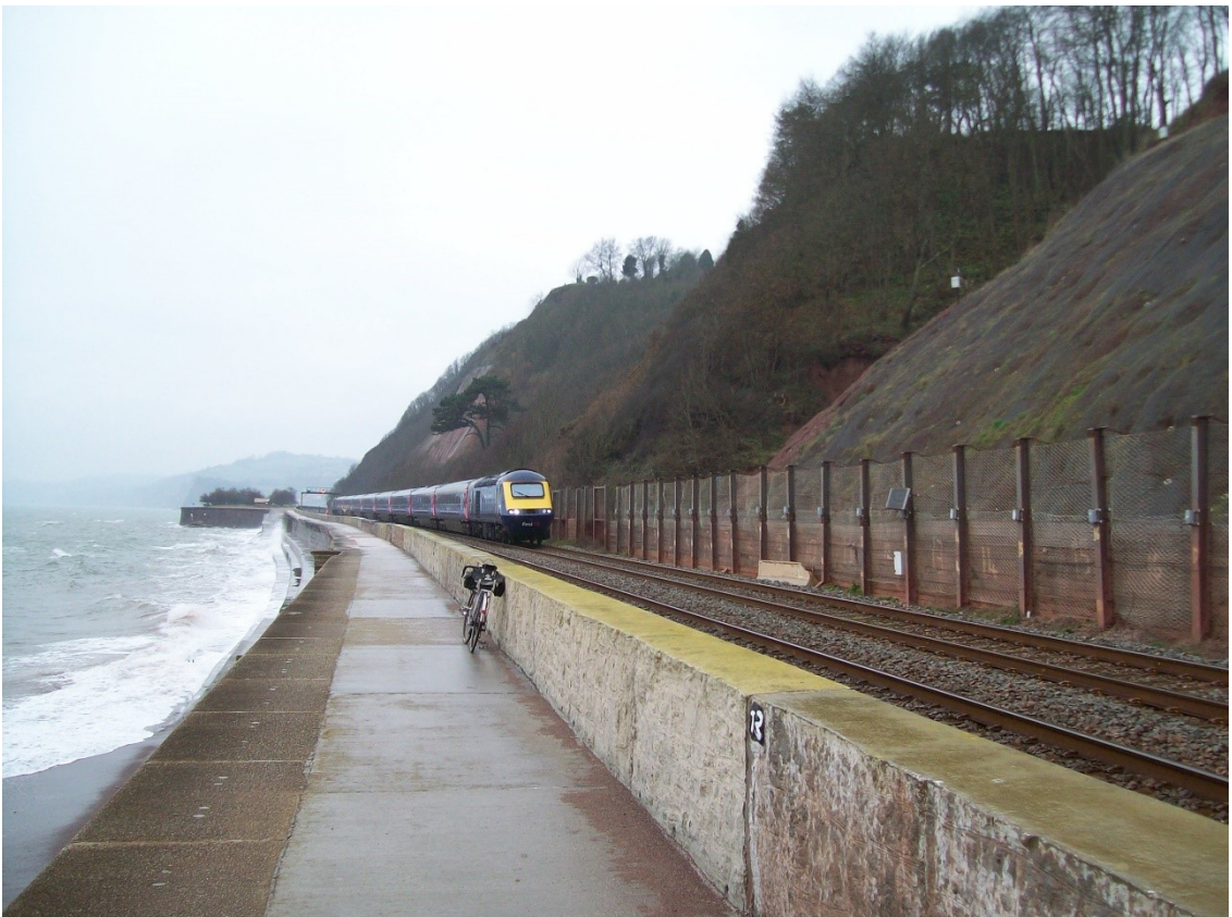
"Tell-tale" devices can be seen attached to the barrier giving some protection from slippage.
