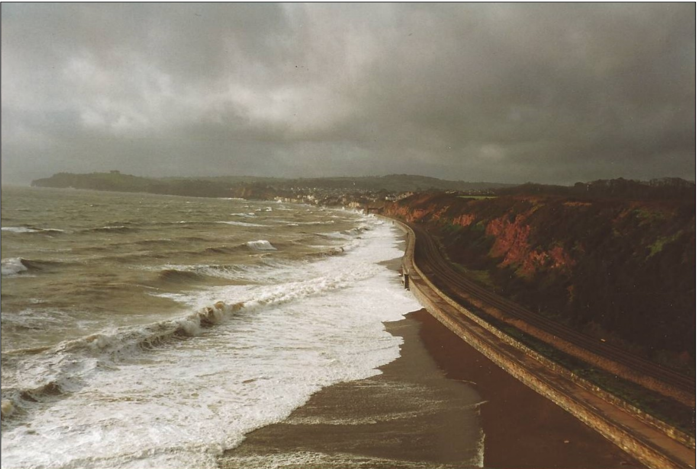
Taken from Langstone Rock on 12th January, 1996. On this day, the Down line was closed because of damage between Dawlish and Teignmouth, and only some trains were using the bi-directional Up line. The service was disrupted for several days on this occasion. The Parson and Clerk can be seen to the extreme left.
