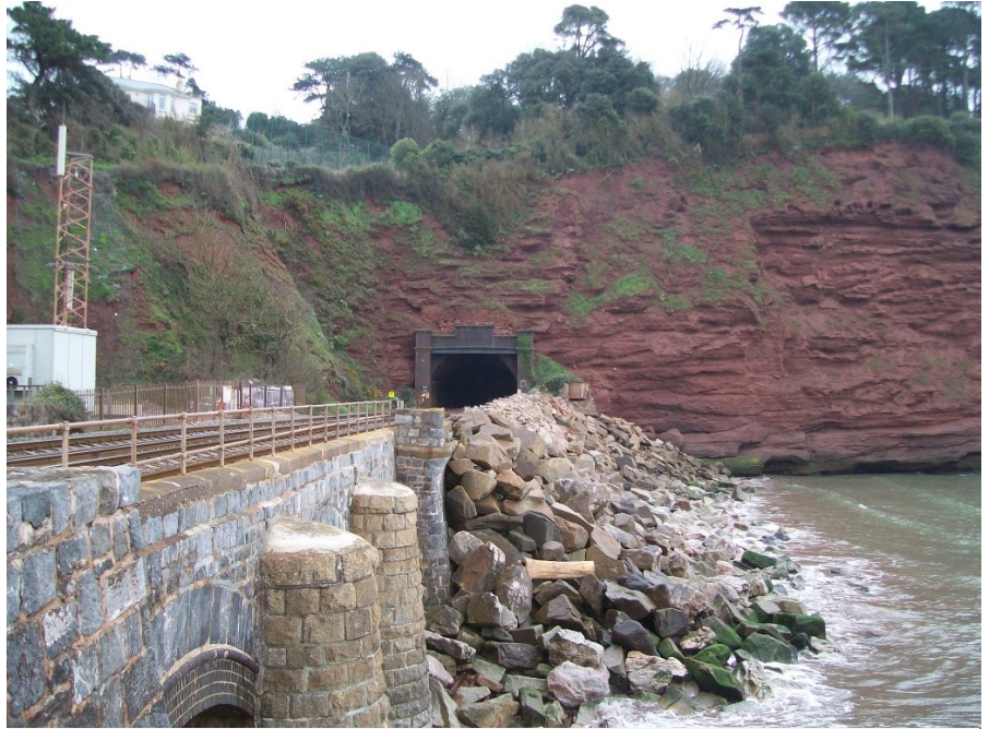
One of the solutions proposed by Network Rail along the length of line where the cliffs are seen to be the greatest threat is a new alignment further out on the foreshore. This would diverge from the existing within Parson's Tunnel and emerge from the cliff seaward of the western portal seen here. It would then run above a new sea wall of modern design nearly all the way to Teignmouth.
