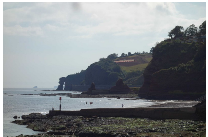
A works compound is being established on top of the cliff, preparatory to the construction of the rockfall shelter at the eastern end of Parson's Tunnel.
