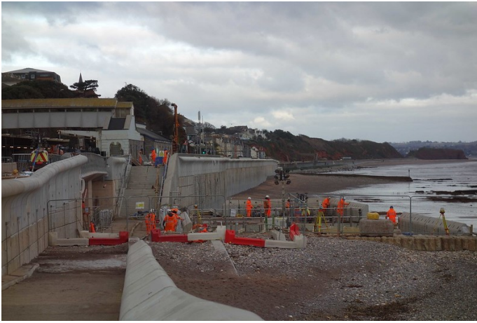
January, 2023: Construction of the new stilling basin is in progress. The new promenade footbridge is in place but not yet open. When the stilling basin is finished, the nine-year, on and off engineer's occupation will be at an end. Unless the 200-year storm occurs.
