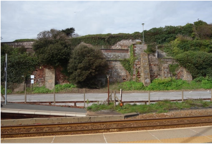
The remains of the atmospheric pumping station at the back of the former goods yard. The stations on either side were Teignmouth and Starcross, where the building survives.
