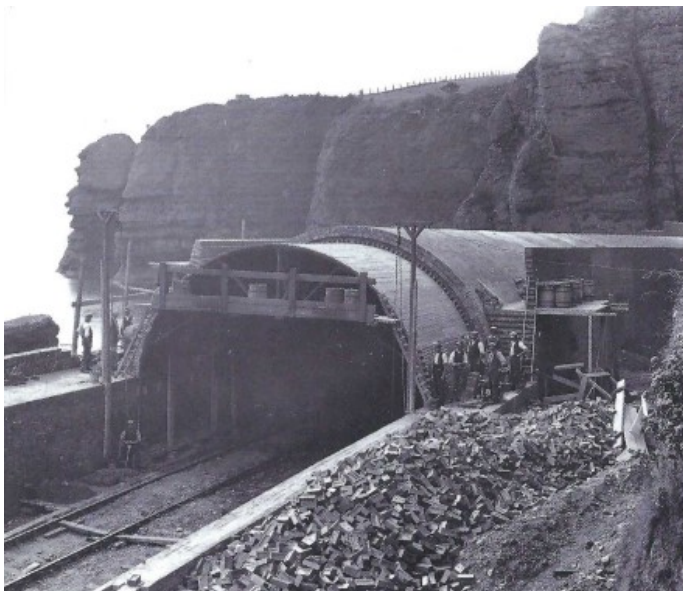
The arch—five rings of brick—was constructed using a shield of bent rails to support the centring. The Parson and Clerk is seen at left.
