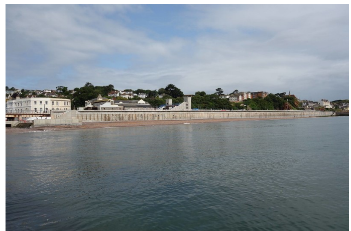
Altogether, there are 164 precast facing panels in this section of the new wall.
