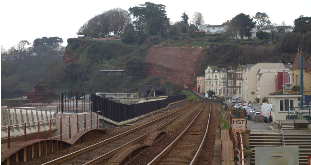
The contractor's men have returned from lunch and can be seen on the cliff above Kennaway Tunnel. In the beginning, there was a very pronounced falling gradient immediately beyond the viaduct in order to meet the agreed height of the rails above Marine Parade. Such a sudden vertical transition would not suit today's 60 m.p.h. line speed.
