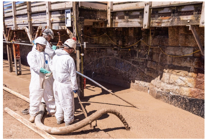
Thousands of tons of this low carbon concrete were used to infill between the new and old walls. Many familiar features were steadily hidden as the level of concrete rose to platform level.
