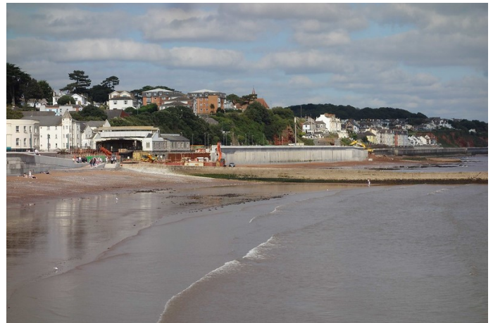
The extent of Phase Two is seen from Boat Cove Breakwater. The piles are still visible in front of the station building. Engineers have now occupied this area almost continually for over seven years.
