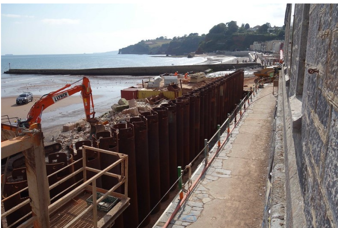
The row of piles, as yet unfaced, continues to the stilling basin. The walkway is still intact, except for the addition of a site safety fence.
