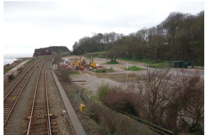
The car park at Dawlish Warren, taken over in 2014 as a works compound, has now very nearly been restored. In the distance is Langstone Rock from where the Teign Valley scout photographed the line on 5th February, 2014, not then knowing that the sea wall had been breached.
