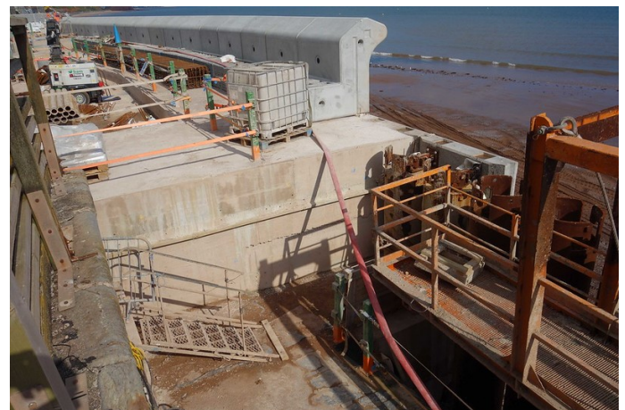
This view provides a good cross section of the work. At left is the original wall at the back of the Down platform, beside the building. Below is the low level walkway, which turned left where the temporary steps are to continue beneath the timber platform. The green posts, below, are on the edge of the walkway. The cylindrical piles, the precast facings and the wave return cappings can all be seen. The space will be filled with mass concrete up to the level of the new walkway.
