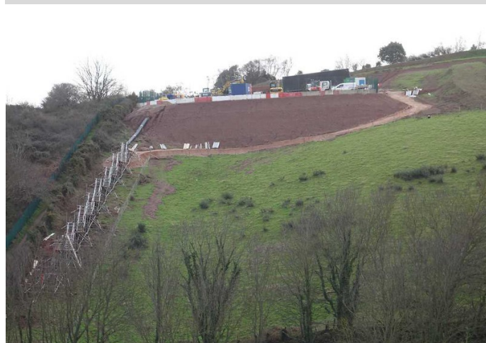
The subsidiary works compound and scaffolding steps under construction, viewed from the coast path. The path, with its precarious steps, continues beside the green fence at left.
