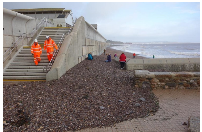
Several hundred tons of beach material had been swept onto the promenade by the stilling basin. Like Beefeaters at the Tower, remnants of the Orange Army seem to be on permanent patrol at Dawlish.
