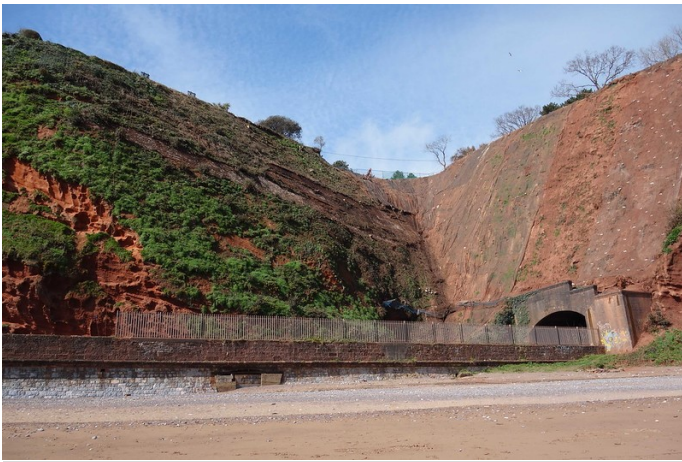
Netting and nailing continues in Coryton's Cove. Lea Mount is at the top of the cliff above the tunnel. The palisade fence is there to deter casual trespass but it makes the area around the tunnel portal very confined.
