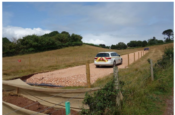
A 12-inch depth of "803" on top of geotextile is more than will be found beneath the ballast of most railways.
