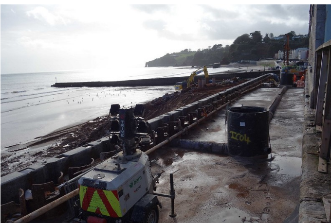
By February, 2022, the old low level walkway had been buried and the piles have been faced. Concrete fill was being built up to the level of the new walkway, indicated by the plastic inspection pit.
