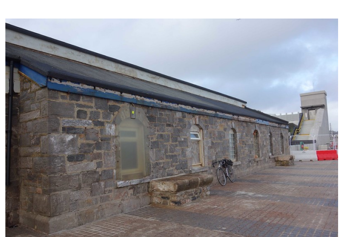
Now protected from the sea and dried out, the Downside building should be ready to undergo repair so that the rooms can be brought back into use.
