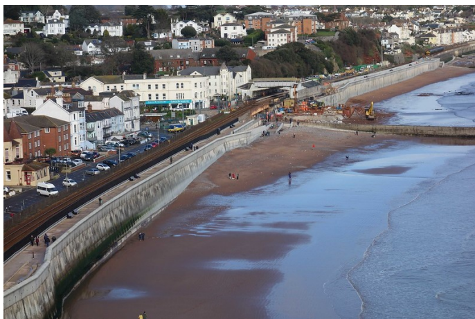
Nearly the whole extent of the new, £80-million wall is seen from Lea Mount. Demolition of the old stilling basin has commenced.
