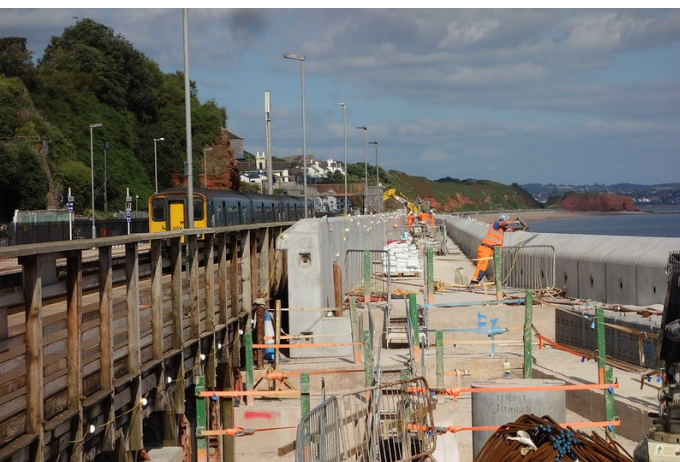
The concrete boundary wall is seen at centre. Planks and boards from the Down platform will never be strewn across the tracks again. The timbers supporting the Down platform are being entombed in concrete. The contractor, BAM Nuttall, with the agreement of Network Rail, chose Hanson's low carbon "RegenGGBS" (Ground Granulated Blast furnace Slag concrete), which, as the name suggests, is a by-product of steelmaking.
