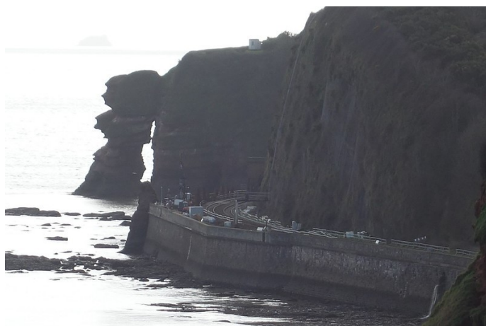
Preparations are being made on a very confined site for the start of construction of the rockfall shelter. Part of the tunnel portal can just be made out. The Parson and Clerk are nicely silhouetted.
