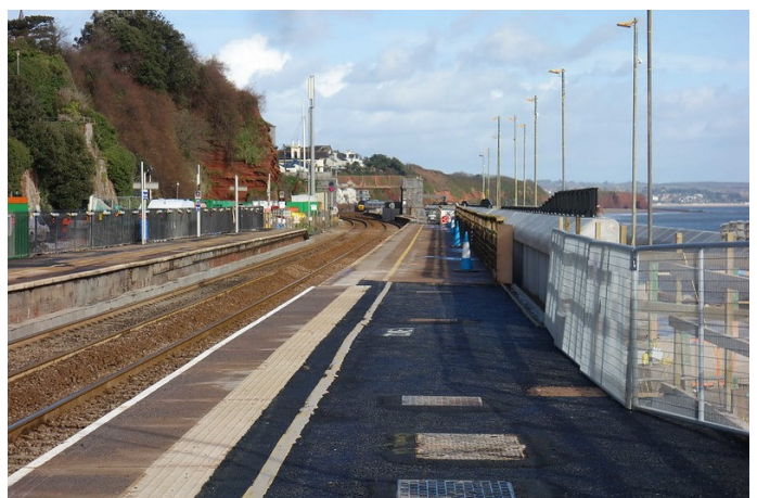
The Down platform had been partly rebuilt and brought up to standard. The remainder of the timber-built platform, beyond, would be removed and the surface made solid. This was where the new footbridge would be built.
