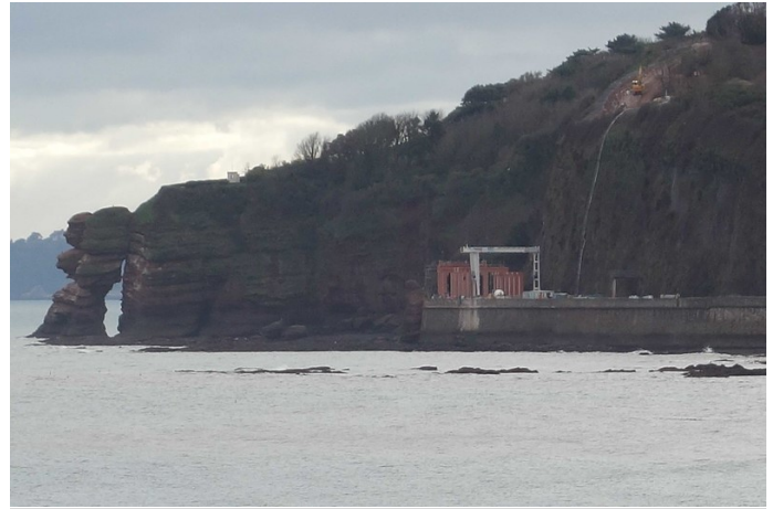
January, 2023: A rail-mounted gantry is being used to position the precast components of the rockfall shelter. Concrete is sent down the pipe seen against the cliff. Viewed from Colonnade Breakwater, about a mile away, a machine seems to be in a perilous position at the top of the cliff.
