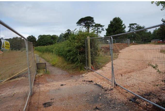
The coast path is crossed by another access road, this one leading to a worksite above the cliff that will be used by the Phase Four contractor, Morgan Sindall.
