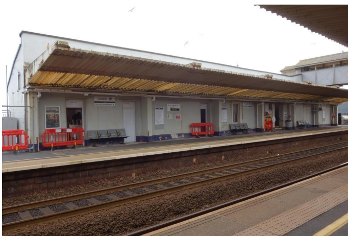
The Downsider building was being refurbished to provide a Waiting Room. There is no exit from the Down platform to the promenade, as it was stated that there would be in the documents, so passengers alighting must cross the bridge and walk around. It is not known whether the emergency exit at the far end of the building can be opened for special events.
