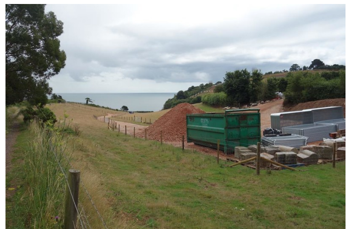
No work can be done in modern times without large compounds and access roads. The land rented from farmers will be made good before being handed back, but it is not known what happens to the thousands of tons of "803" which is used. Here, preparations are being made for the cliff nailing and netting contract, separate from the tunnel work.
