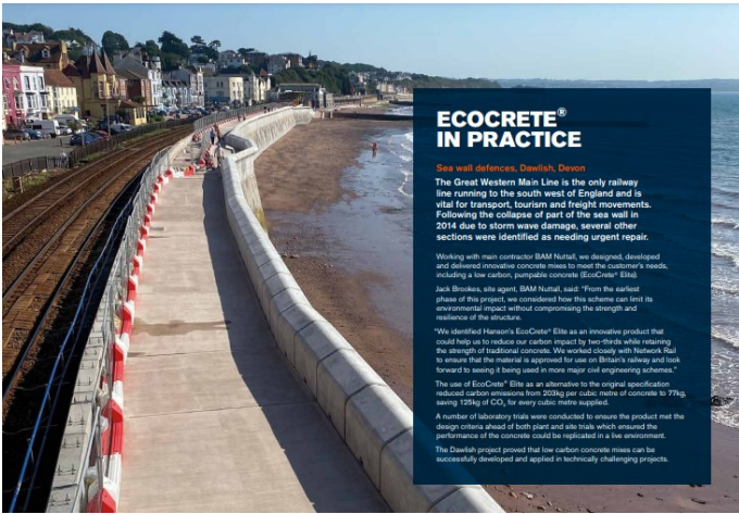
Working with main contractor BAM Nuttall, Heidelberg Materials, formerly Hanson, designed, developed and delivered innovative concrete mixes, including a low carbon, pumpable concrete (EcoCrete® Elite).
