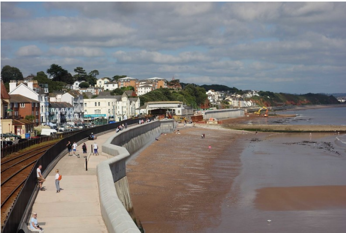
In September, 2021, work is continuing on the wall protecting the station, with most of the precast concrete facings in place and the recurve units above. When £80-million has been spent, there will be a high level walkway from Dawlish Warren to Kennaway Tunnel.
