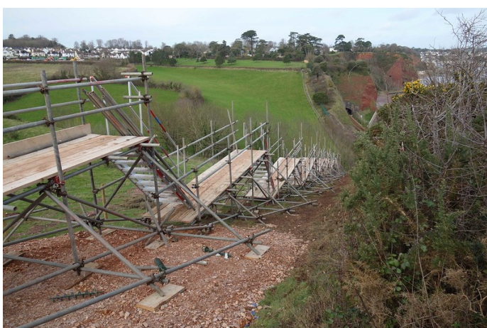
This scaffolding stairway was a major structure in itself: flights of steps to allow workmen to pass safely from the subsidiary works compound above to the work site at track level. Installing a lift beside the cliff, like the ones attached to tall buildings under construction, must have been ruled out. The houses at top left are on the Dawlish to Teignmouth turnpike. The coast path follows the hedge at the top.
