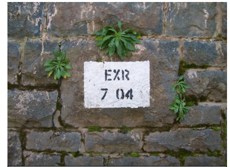
The identification mark on the ruins of Greenwall Lane Bridge, seven miles and four chains from Exeter Railway Junction. Judged as unsafe, the bridge was demolished in 2013 at a cost of nearly £100,000.
