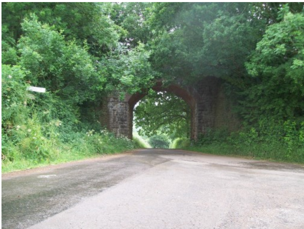
Now heading south-west, the line passes over Sminhay Bridge, where it is clear that the engineer has realigned the roads to make for less expensive construction.
