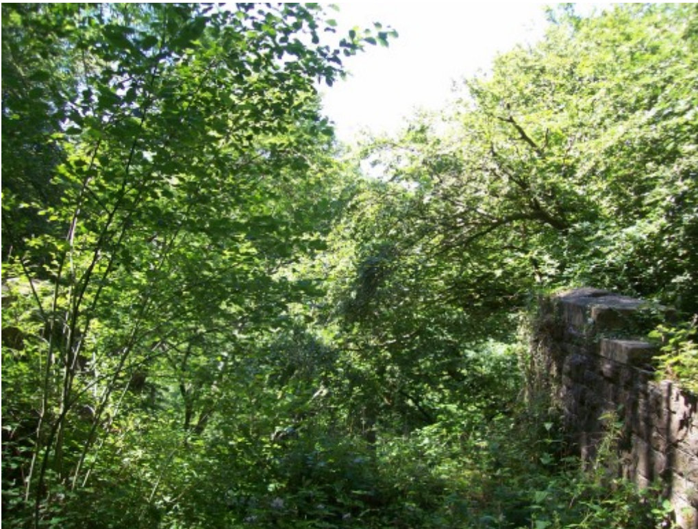
Taken from the abutment at the Taunton end, there is a void once spanned by steel. The first pier can just be glimpsed through the foliage.
