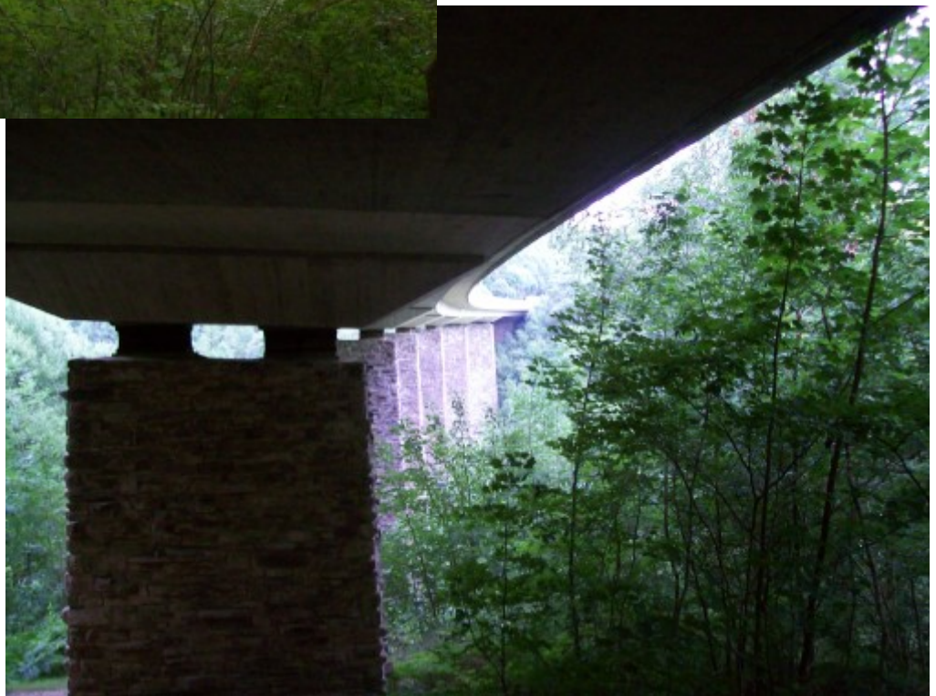
At the Barnstaple end of the viaduct, the immediate new pier is followed by the five originals, now raised .
