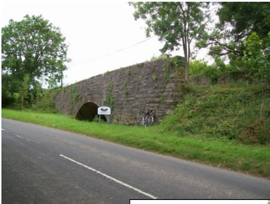
The bridge which carried the B3190 over the Barnstaple Branch near Morebath Junction is now partly filled in and bypassed.
