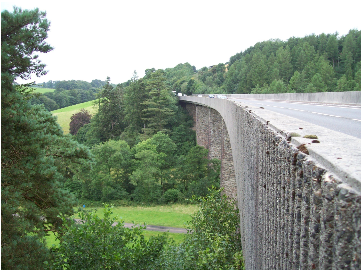
Unseen by the myopic motorist are the slender masonry piers which carried the single line of rails of the Barnstaple Branch across the Bray Valley. The river is amongst the trees beyond the track. Between them was M.P. 200.
