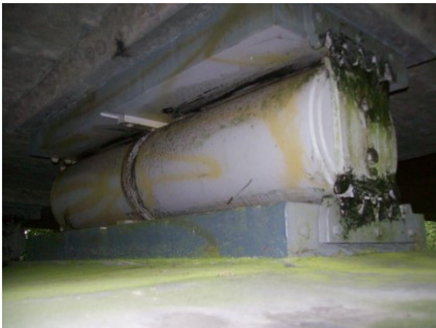
One of the two bearings at the top of each pier. With the darkening skies over Barum, there wasn't likely to be any movement on the day this was taken.
