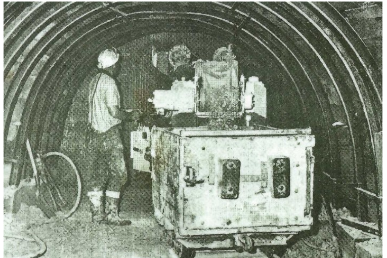
A working face in one of Watts, Blake, Bearne & Company's Kingsteignton mines in the 1970s, showing a Westphalia boom-cutter loader filling a single 12 cwt. Truck. This would have been man-propelled back to the main haulage adit.
